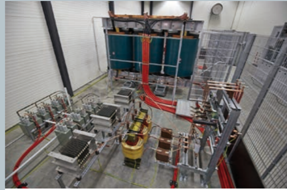
Filter installations at the grid emulator part of LORC's nacelle test facilities.
