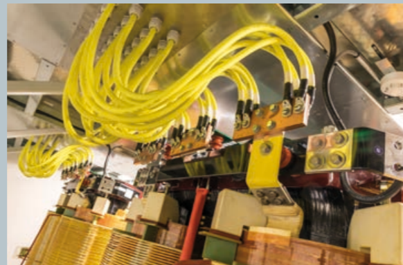
Transformer-converter connections at the LORC HALT test facility.
