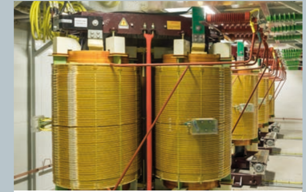
The transformer hall at the LORC HALT test facility.
