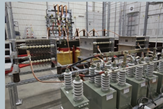
Filter installations at the grid emulator part of LORC's nacelle test facilities.
