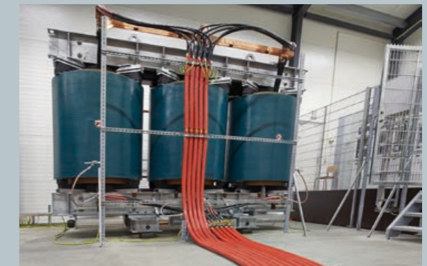
The transformer hall at one of LORC's megawatt nacelle test facilities.
